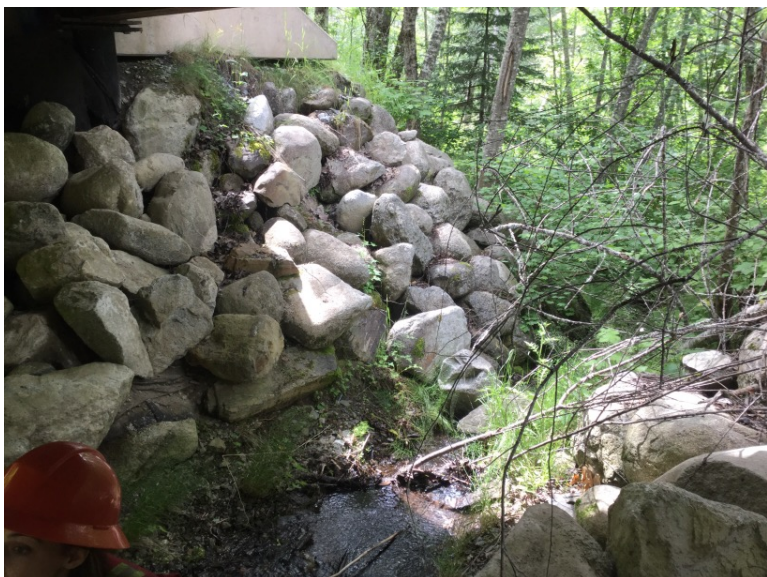
Riprap condition at downstream left bank
